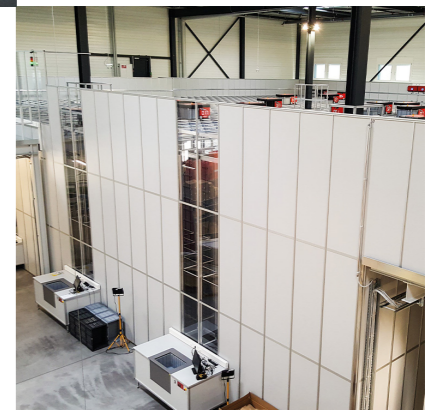
With the autostore at the L.I.T. Warehouse in the Bremen GVZ, the company is taking an important step towards digitalization and automation.
